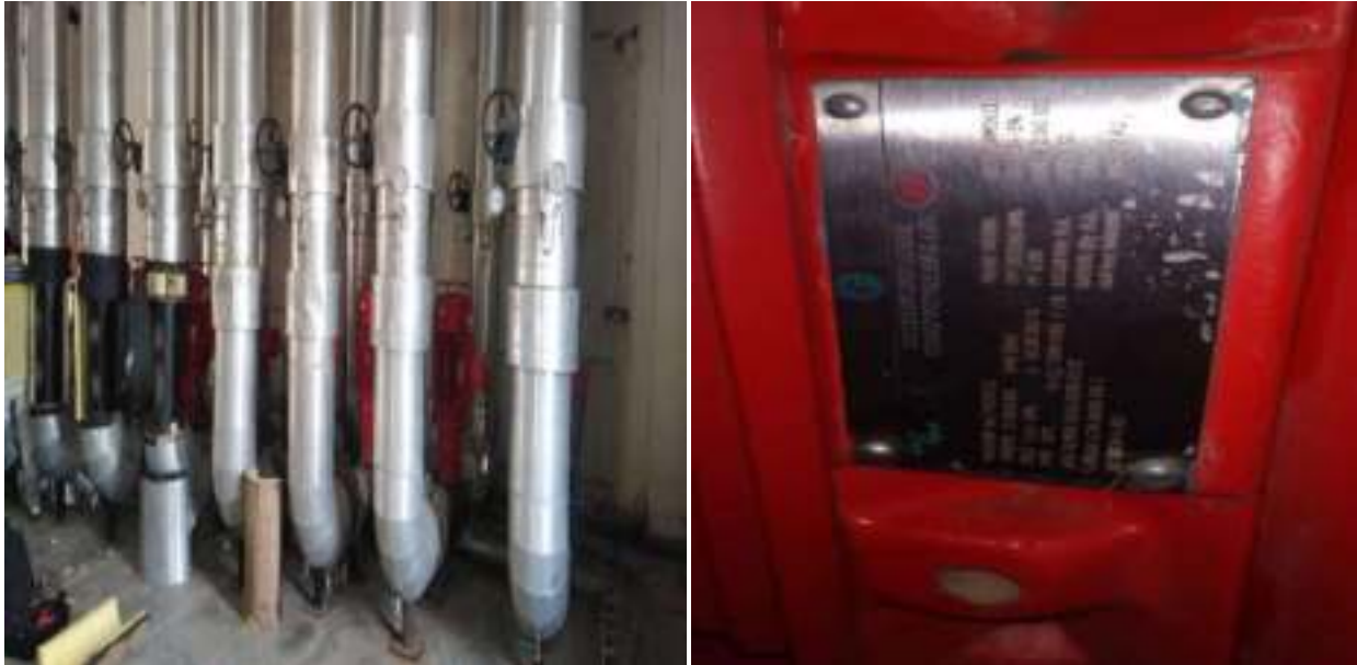
Figure 7:Chilled water pumps
