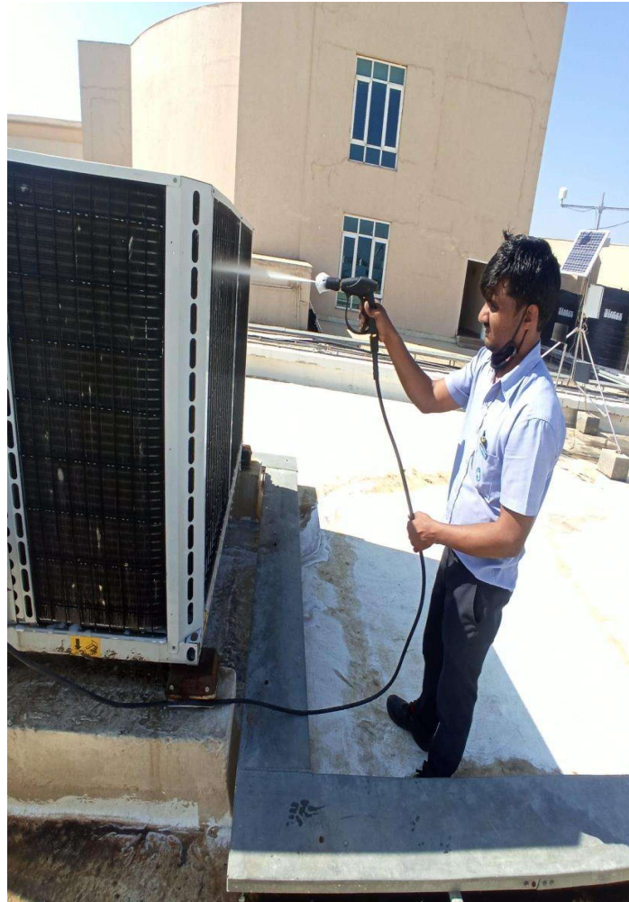
Chiller Cleaning – Right Wing
